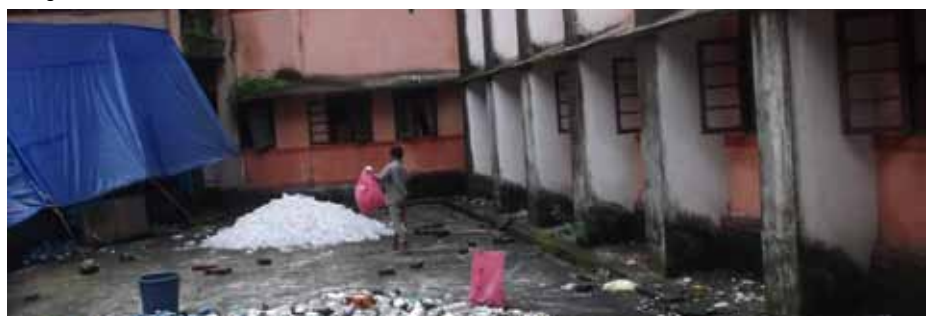
Piles of drug and saline bottles, and the dilapidated hospital structure.
